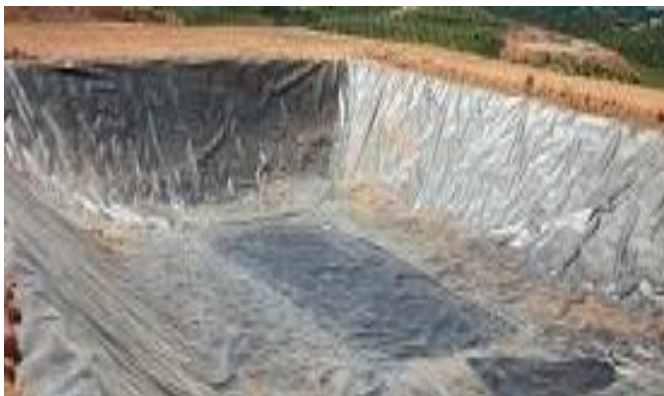
Figure 6. Rainwater reservoir with plastic lining
