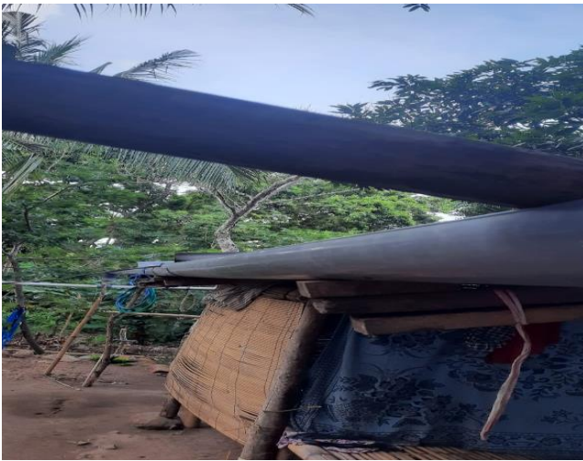
Figure 10. Rainwater catchment network from PVC pipes
