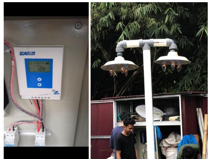
Figure 4. Commissioning test of PLTS system
