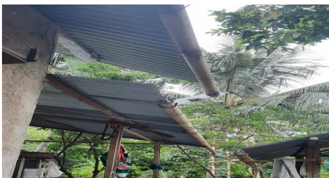
Figure 2. Rainwater Capture System from the Roof of the Building
